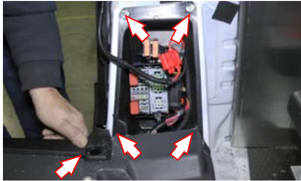
Distribution panel and stepwell screws
