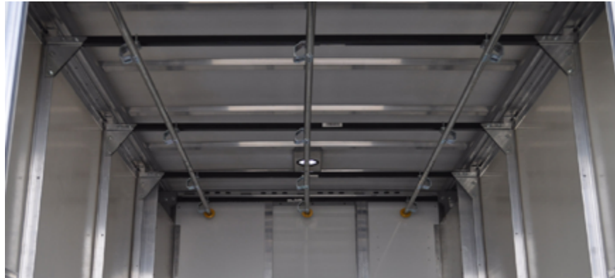
Linen (pipe rack) package
